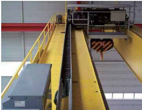
拖链系统可安装在起重机大梁上
